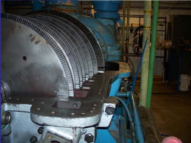
This small industrial turbine turns a chiller.
